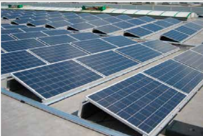
More than 4,000 solar panels provide our factories with electricity
